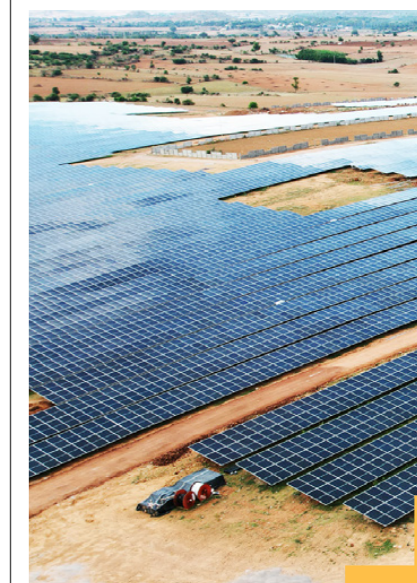
Actual site of 42.9 MW renewable energy project at Kudligi Taluk, Vijayanagara District, Karnataka
